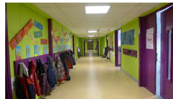
T8 fluorescents 36Wx2 in corridor in primary building
