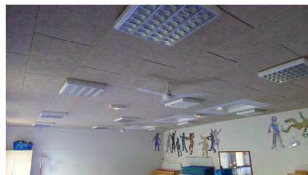
T8 Fluorescents 18Wx4 in classroom in pre-schol
